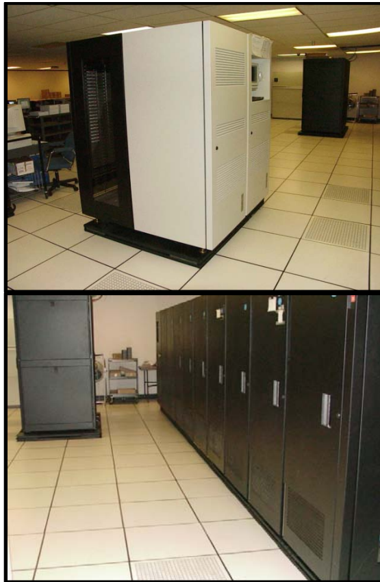
Non-structural seismic mitigation for State Controller's Office
